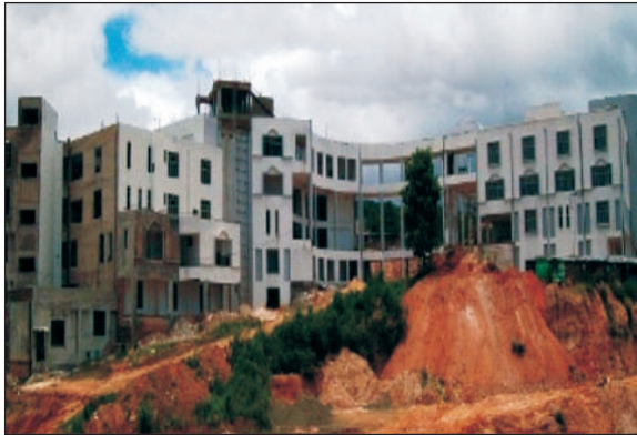
Construction of Hospital Complex for North Eastern Institute of Ayurveda & Homeopathy (NEIAH), Shillong, Meghalaya
